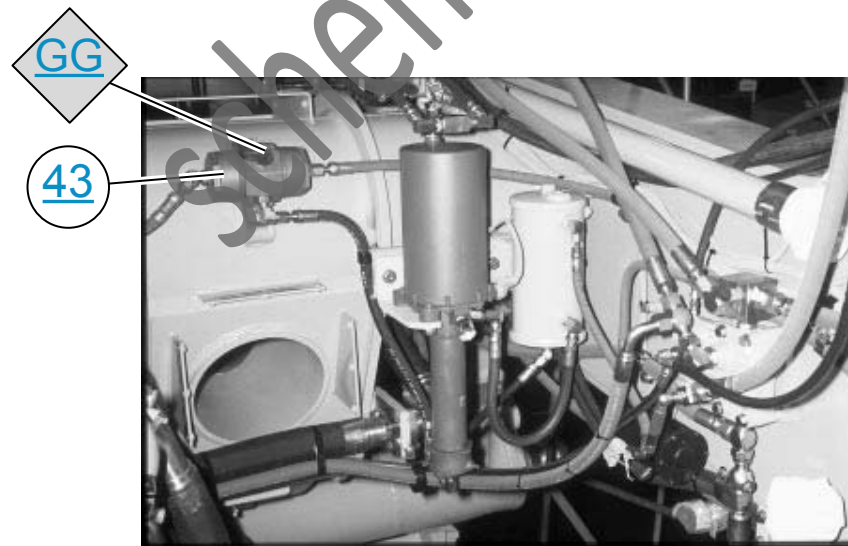
Oil Makeup Tank Area
